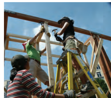
Top+Middle: Gullwing Porch at Community Forge: Eddie Fischer+Owen Haft (B.Arch '21), Ryan Smerker (M.Arch '21)
